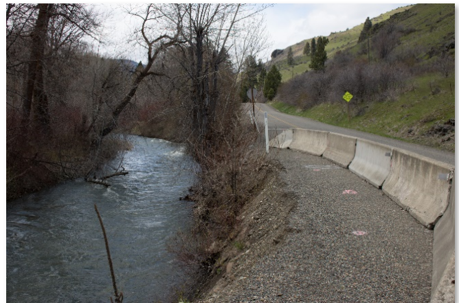
An example of maintenance needs on County roads.
