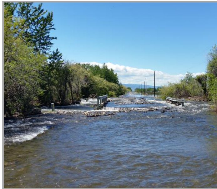
Flood event of 2017; overtopping bridge.
