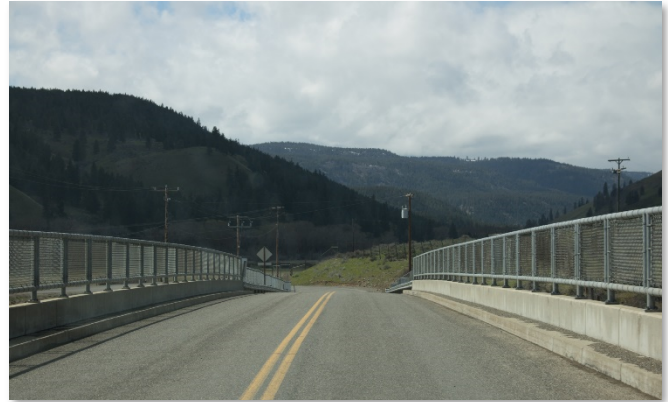
Some bridges may not show visible signs of wear but proper maintenance is necessary to keep them in good repair.
