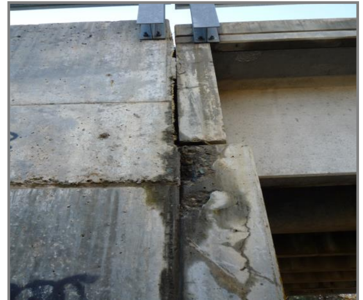
Joint damage visible at inspection
